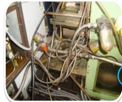
Figure 5: Wires and Pipes not routed
